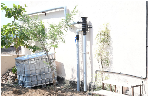
Composters installed at Chandus
